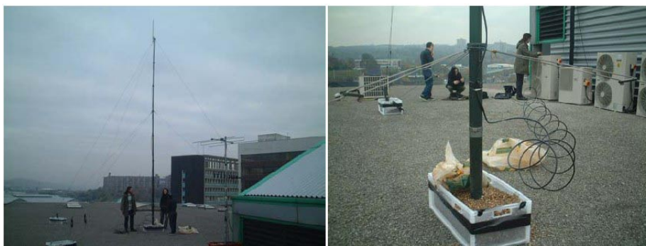
Fig. 5. Eight-meter high-power omni mast
